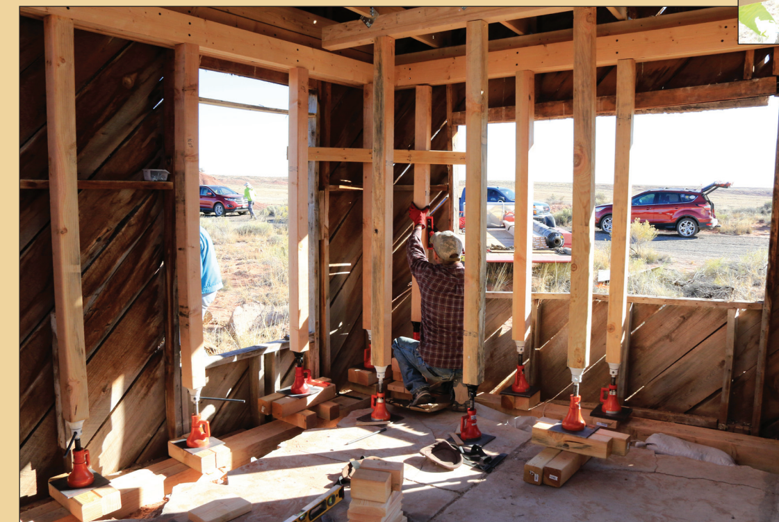
A crew member uses a level on a jack post. If even slightly off, the screw jack beneath the post could roll over under the building's weight.
