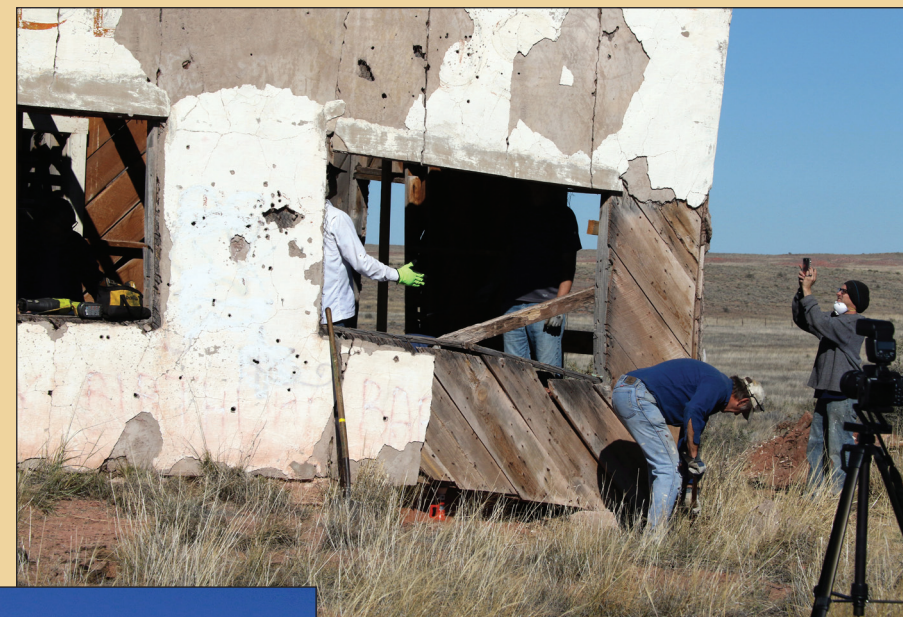
A screw jack is placed under the dangerously sagging southeast corner to provide temporary support.
