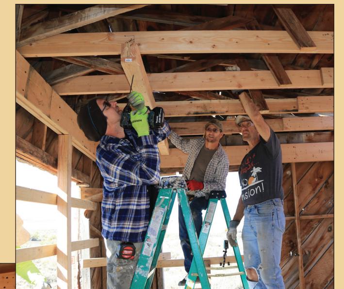
Crew members install a beam in preparation for raising the building's southwest corner.
